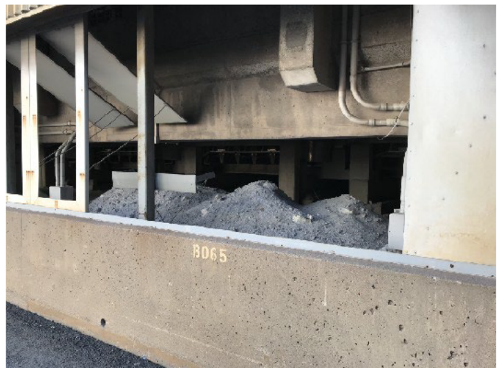
(photo 6) IMG_0673.JPG Poussière de bain vis ble sous les hall B et C
